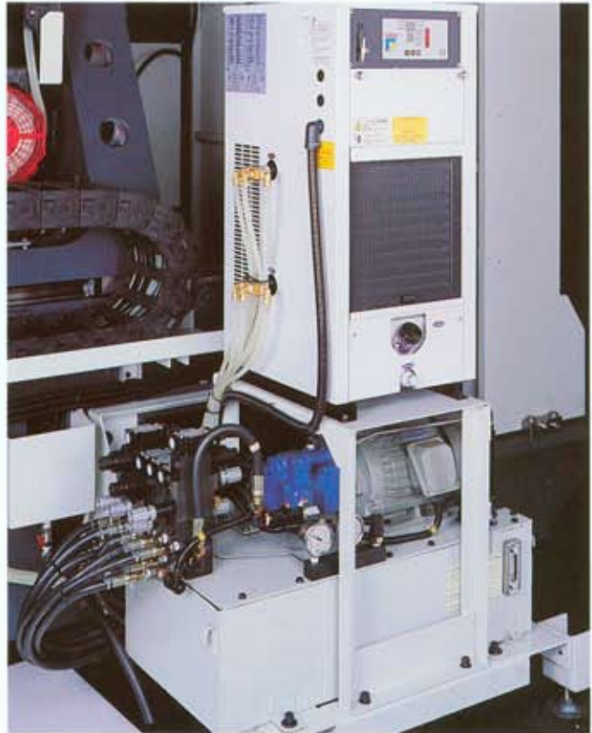
Piping centralized (Hydraulic system)
